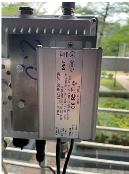
Figure 8 power adapter installation
